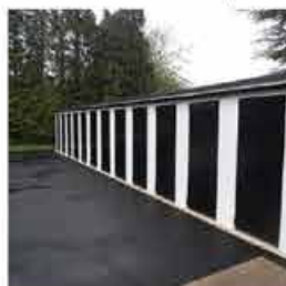
Demolition and Construction of New Sheds. Grade II Listed Site. Contract Value £30,000.
