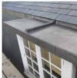
Old Street, London. Roof Replacement Project. 5 Grade II Listed Terrace Blocks of Flats. Contract Value £150,000.
